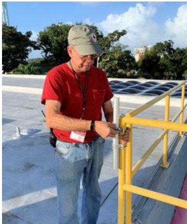
Puerto Rico Section Manager Oscar Resto, KP4RF, installs an antenna at Red Cross Headquarters in San Juan.
